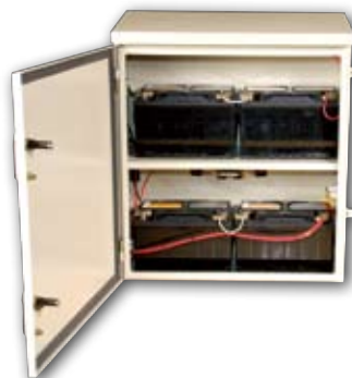
24 Hour backup solution with extended batteries
